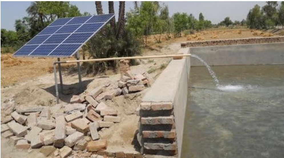
Figure 3. Solar collector through which the irrigation pump is powered
