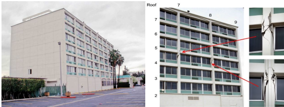
Figure 2. View of the hotel “Holiday Inn” in Van Nuys from North-East Figure 3. Post-earthquake view of in Van Nuys damaged columns
