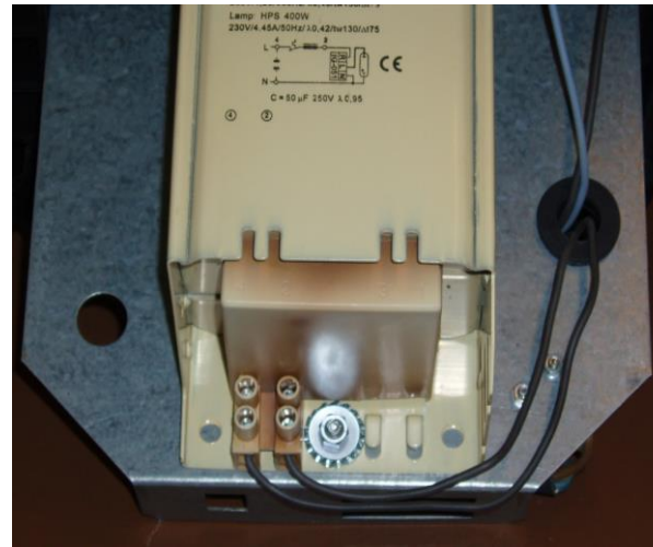
Fig. 2 A choke showing a change in the color of the cover due to increased temperature
